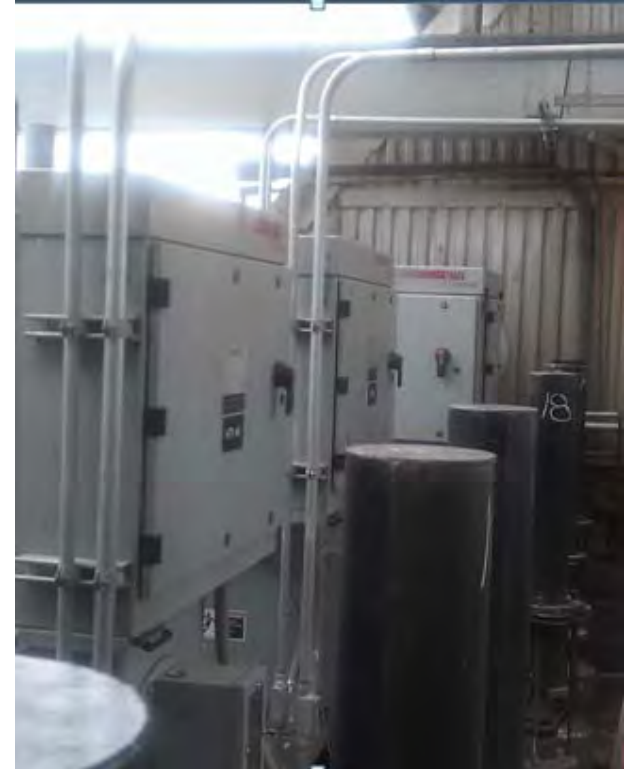
Overhead Cable Tray will Limit HV Unit Replacements
